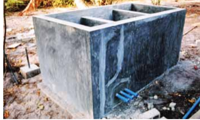
Sea water sedimentation tank before desalination.
